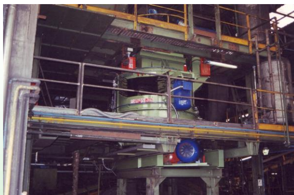
AER-A-MIX 100/270 in impianto esistente. AER-A-MIX 100/270 into existing sand plant
